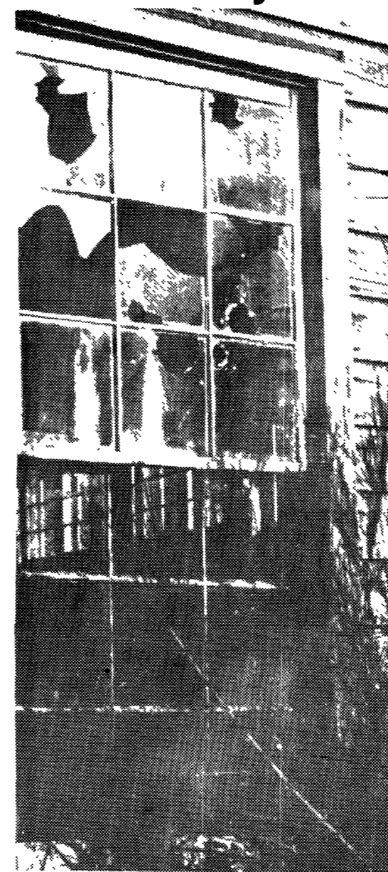
Broken windows are common here on the Quillayute.
